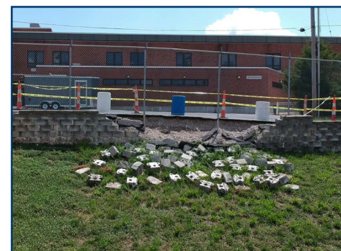
A portion of a retaining wall near the Oakville High School football stadium collapsed during the spring. Crews replaced and reinforced that wall over the summer.
