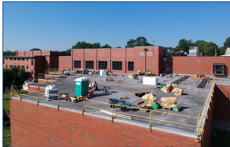
Crews replaced large portions of the roof at both Bernard Middle School and Mehlville High School, pictured above, this summer.
