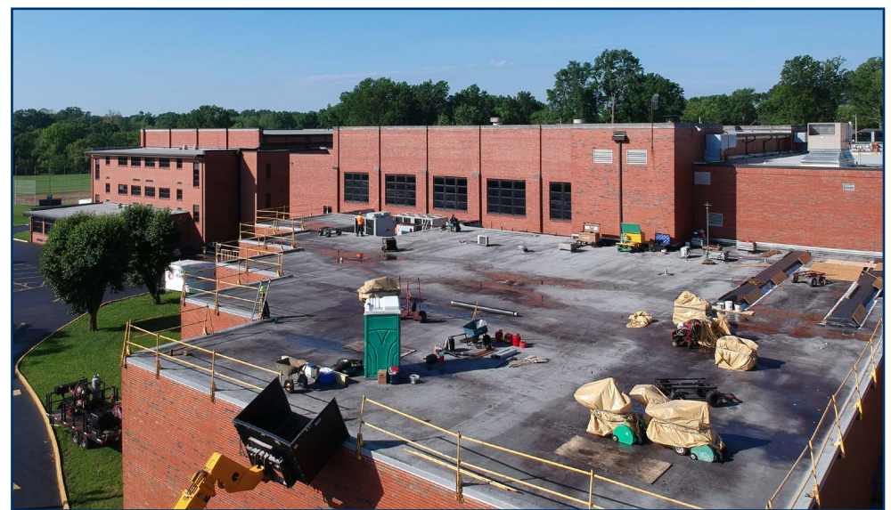
Workers got an early start on the roof replacement of the Mehlville High School library. Both Mehlville High School and Bernard Middle School will receive roof replacements.
